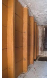
plafond in gang
